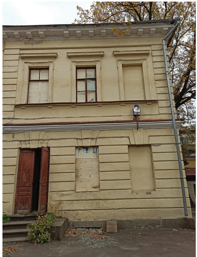
Fig. 5. Broken backyard windows temporarily boarded with plywood and cardboard
