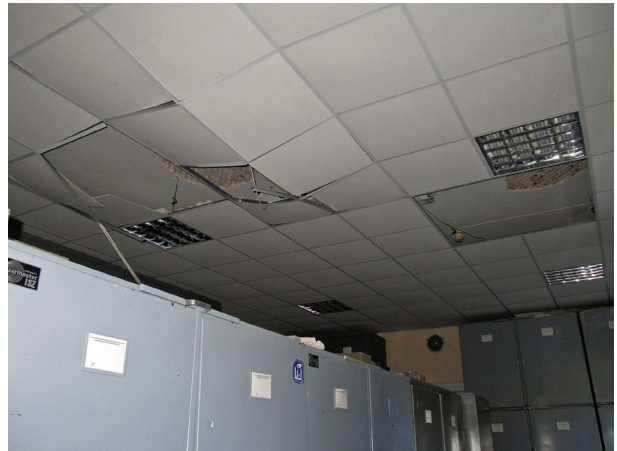
Fig. 3. The damaged ceiling in the Lesser Herbarium Hall
