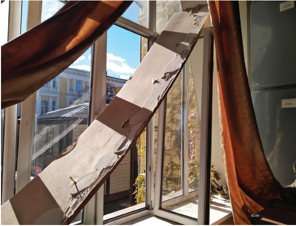
Fig. 1. A damaged panorama window in the Main Conference/Herbarium Hall
